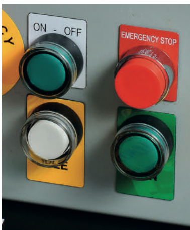
Control panel labels
